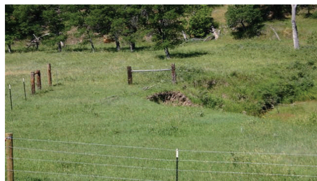
Fencing project to prevent direct access to a riparian area and provide vegetative buffer along the water body
